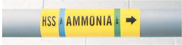
A uniform method of pipe identification, such as this one utilizing IIAR Pipe Markers, helps create a safer, more productive work environment.
